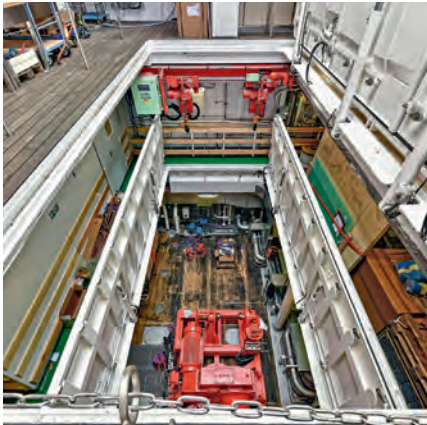
Single girder overhead crane for hangar
